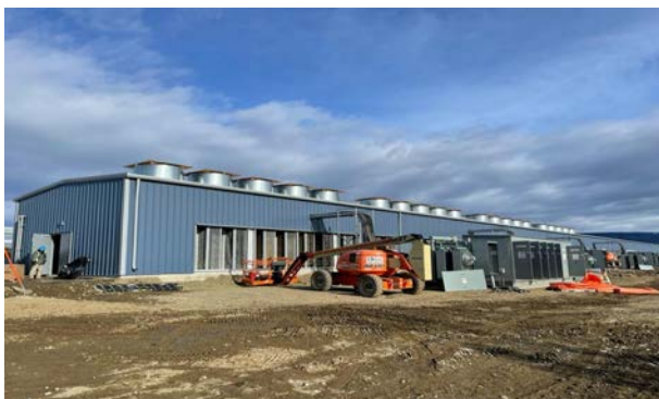
First 20MW data center
