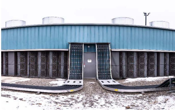
Specialized data center at Canal Flats (0.8 EH/s, 30MW)
