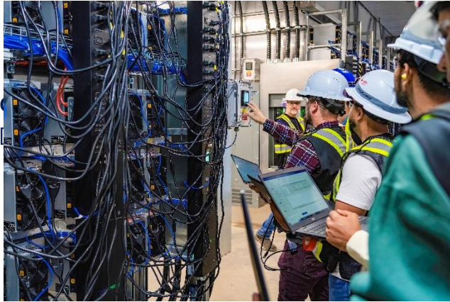
Prince George – technicians energizing ASICs during commissioning
