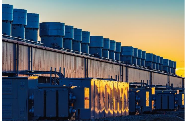
Prince George – fully commissioned
