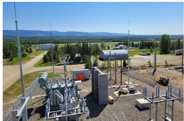
Mackenzie – all major electrical equipment installed in substation
