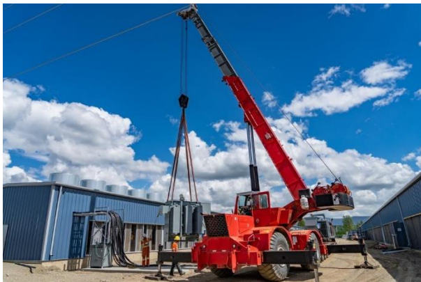
Mackenzie – medium voltage transformer placement
